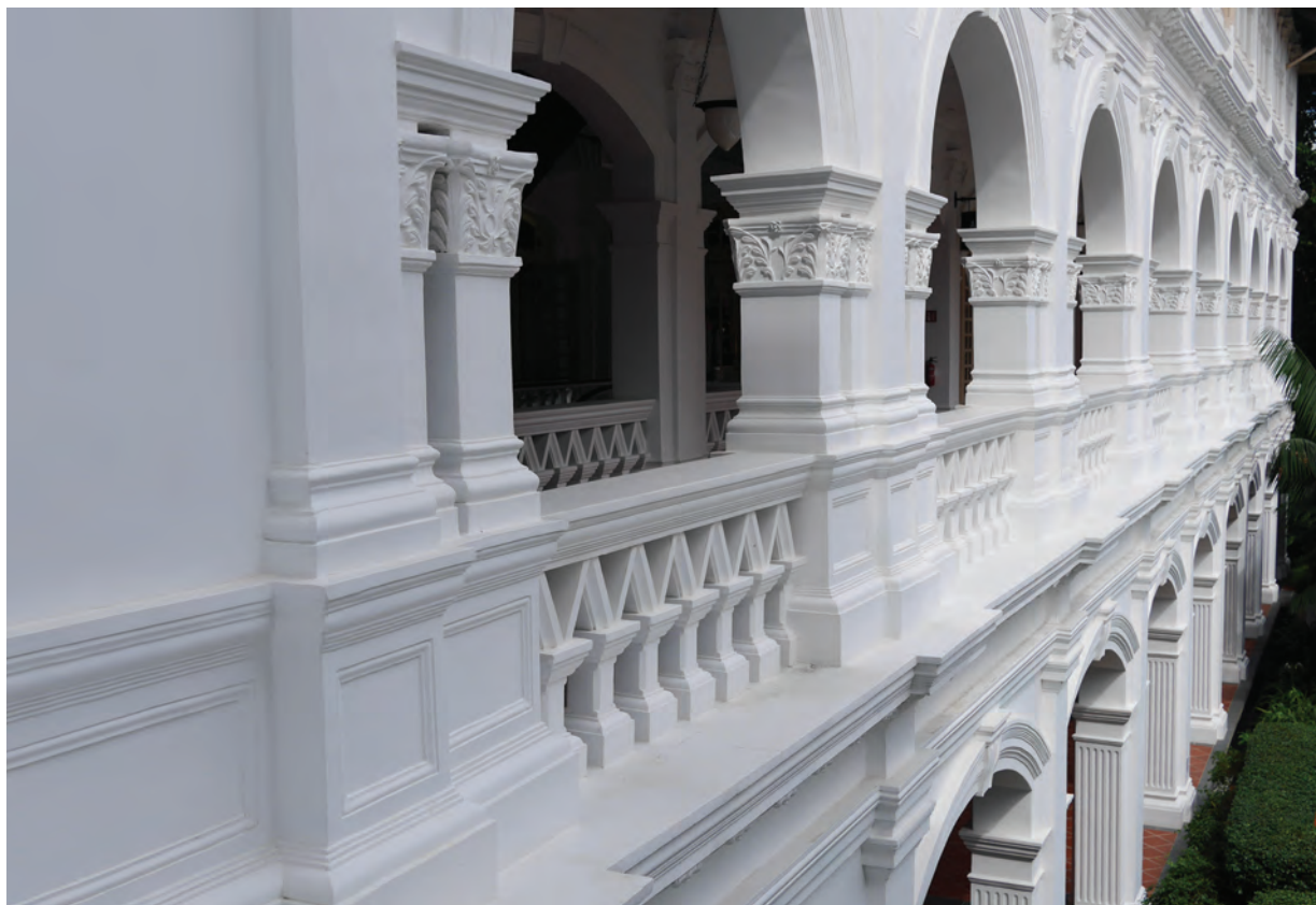
LEFT: The balustrades were restored using Mape-Antique Intonaco NHL base render, which is ideal for application on masonry in historic buildings.
