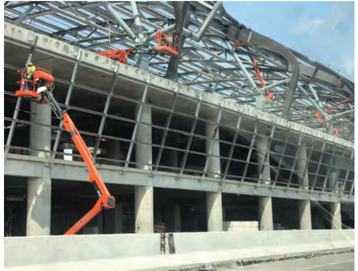
ABOVE AND BELOW LEFT: Dingli’s aerial work platforms being used on the Suvarnabhumi International Airport project in Bangkok, Thailand.
