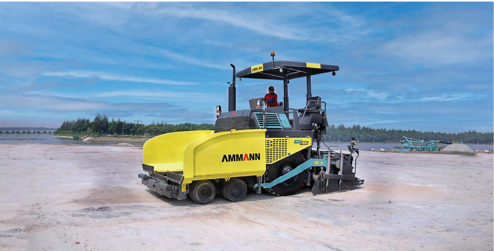
TOP AND ABOVE: An Ammann AFW 500 asphalt paver works at widths up to 5 m, helping NDE Readymix to deliver the project on time.
